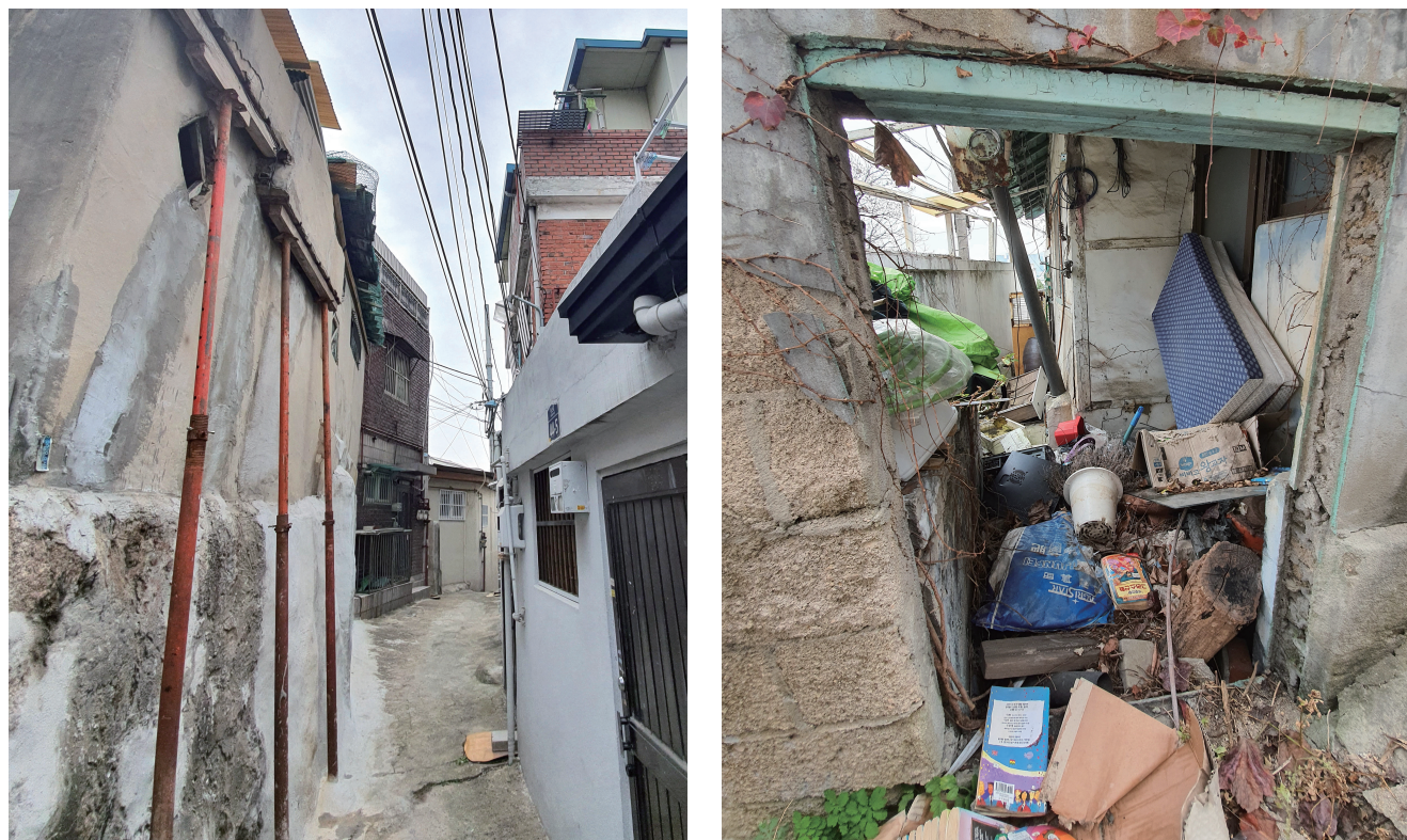
Figure 2. Safety risks and hygienic issues caused by collapse of neglected vacant houses
