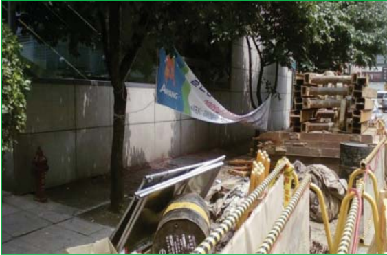
Figure 2: Path Obstructed by Construction
