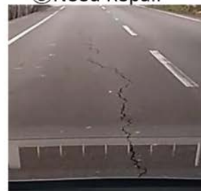
③ Need Repair
